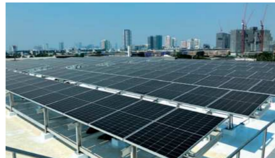
Photovoltaic power generation equipment installed on the roof of the new building of Yuasa Trading (Thailand) Co., Ltd., our group company
